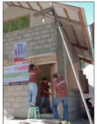
LOTIFF Engineers installing the last piece before turning over the unit. Involved are Engr. Mikko Lora, Engr. John Laborada, Jonathan Uy.
